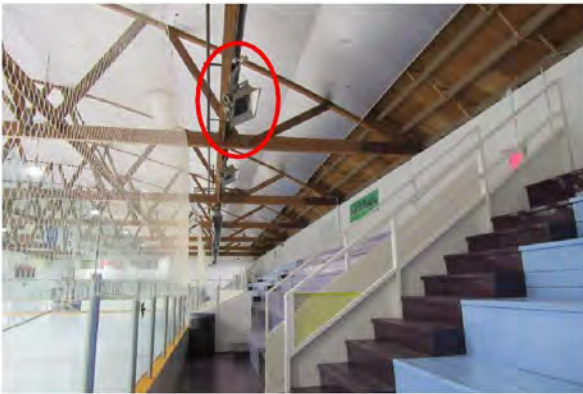
Photo #M7: Overhead electric radiant heaters.
