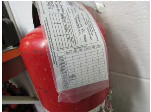
Photo #M12: ABC fire extinguisher.
