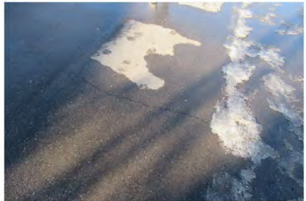
Photo #A2: Asphalt Cracks in parking lot.
