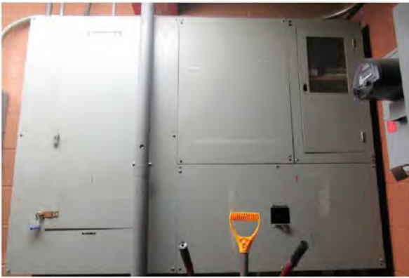
Photo #E3: Central distribution panel/switchgear.
