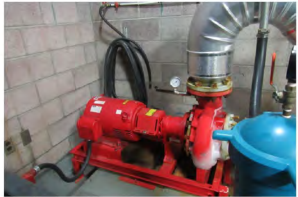
Photo #M16: Brine Pump.
