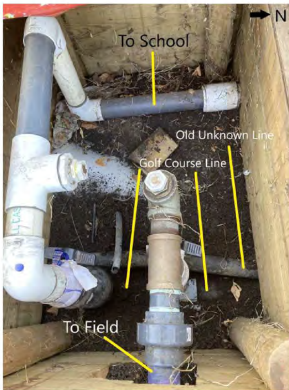
*Matthew Halton Main Valve Box (2022)
