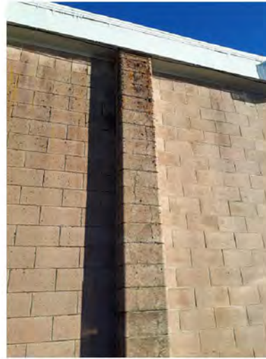
Photo #S6: Cracks in pier of the exterior CMU wall.
