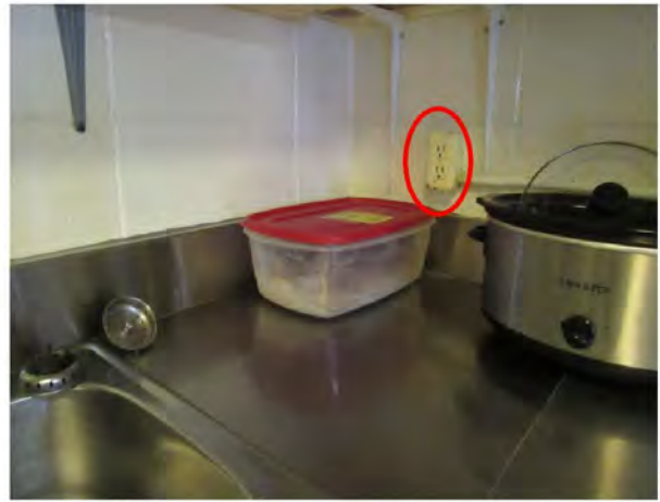
Photo #E6: Non GFCI receptacle found within 1 meter of a sink.
