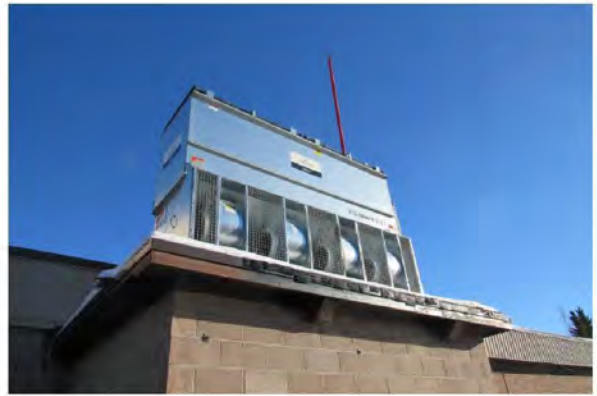
Photo #M14: Cooling tower for ice plant.
