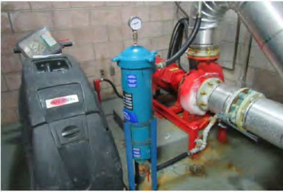
Photo #M17: Brine pressure gauge.
