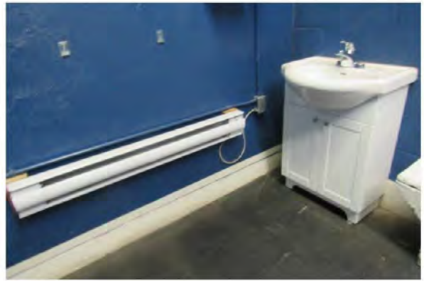
Photo #M6: Hydronic baseboard heater.
