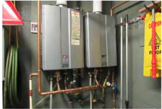
Photo #M8: RINNAI instant hot water heaters.
