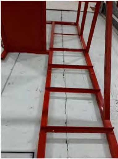
Photo #S3: Vertical joint separation in CMU wall.
