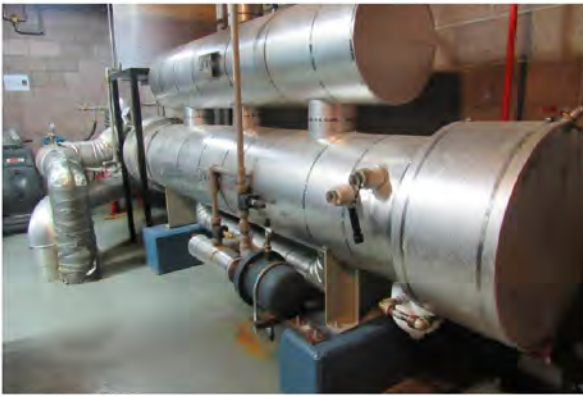
Photo #M13: Ice plant chiller/heat exchanger.
