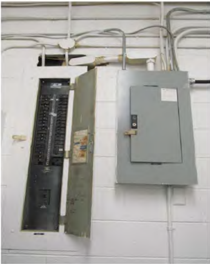
Photo #E5: Subpanels located in referee room.
