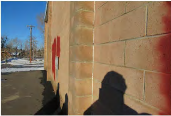
Photo #A7: Disconnected Joint Sealers on the exterior wall.
