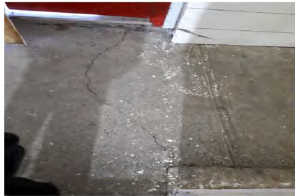
Photo #S2: Crack in slab-on-grade under the seating area.
