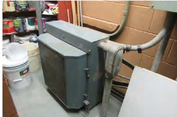
Photo #E2: Interior transformer.
