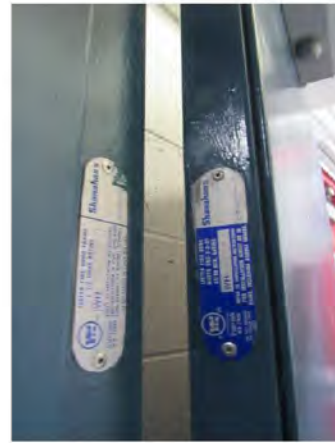
Photo #A16: Interior fire rated door.
