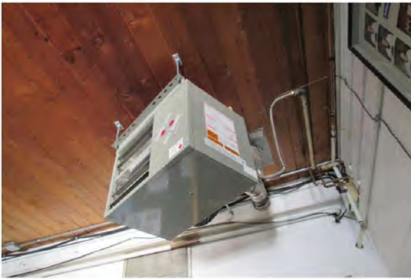
Photo #M5: Ceiling mounted radiant heater.
