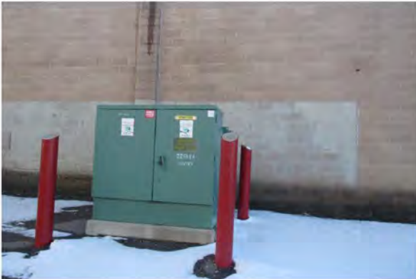
Photo #E1: On site electrical transformer.
