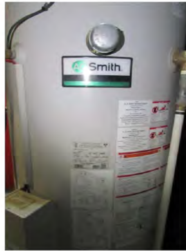
Photo #M10: AO Smith water heater.
