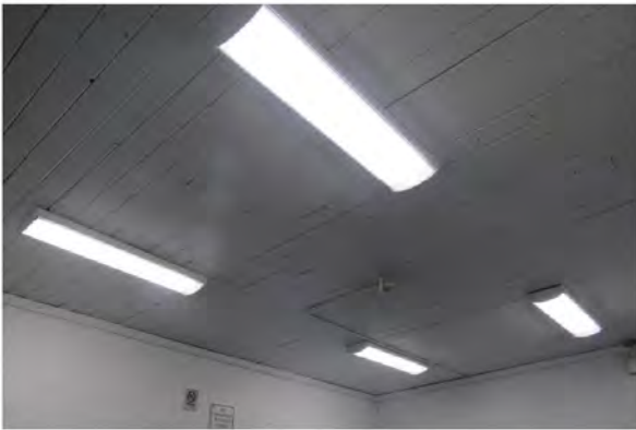
Photo #E7: Ceiling mounted fluorescent lights.
