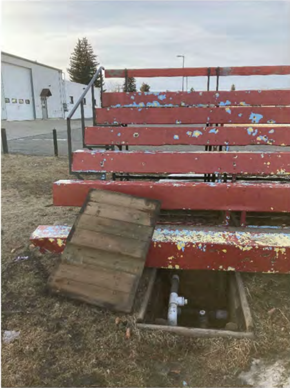
*Matthew Halton Main Valve Box (2022)
