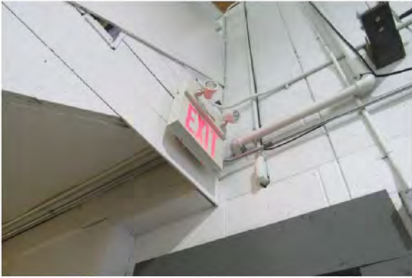
Photo #E9: Exit and emergency lighting.
