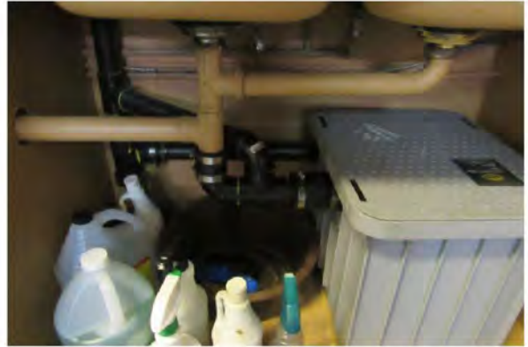
Photo #M2: Grease trap and piping.
