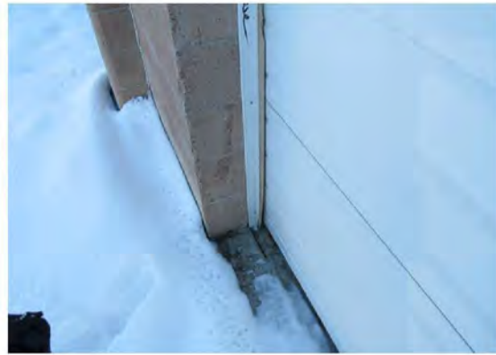
Photo #A8: Improper sealant (weather stripping) shown at the overhead door on the rear of the building.
